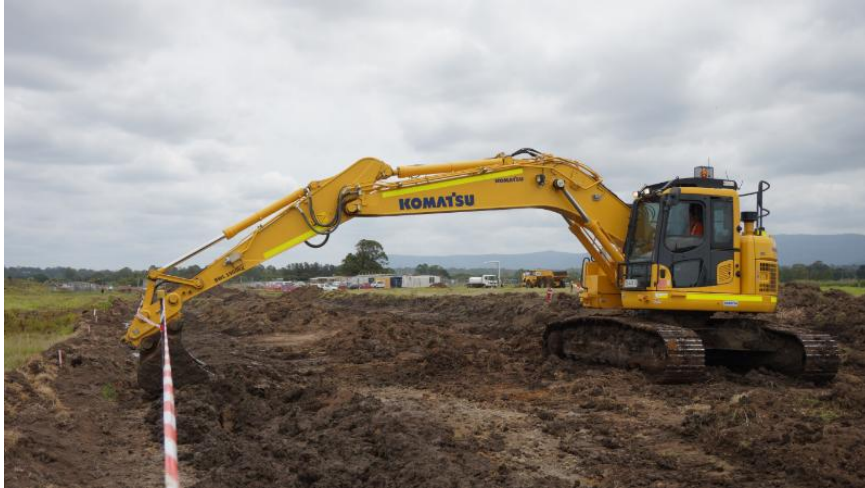
Backfilling operation followed by forming bunds on the top of the slurry wall
